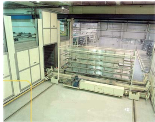
Automated trolley in a floor oven design
