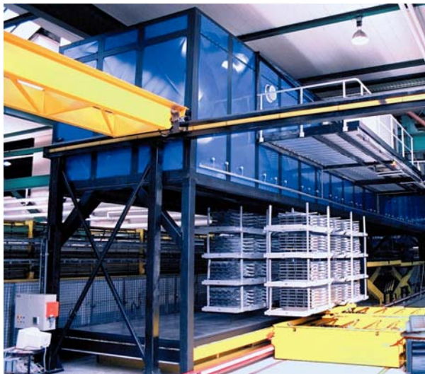
Loading of a vertical chamber oven
